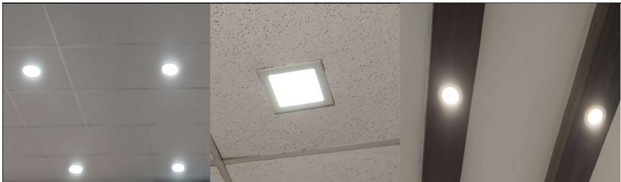
Example of Energy Efficient Appliances Usage :Use of LED lighting
