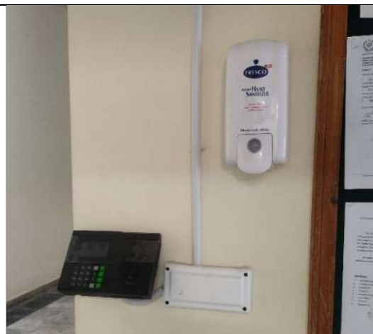
Sanitizers/Disinfection units installed at all buildings entrances
