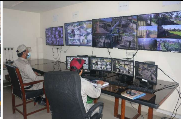
4. Security Control rooms
