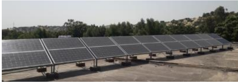
Solar Panels installed at main campus and some regional campuses
