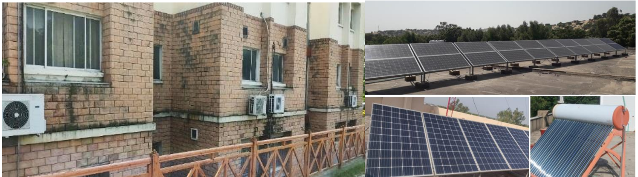
Energy efficient inverters (Combined Cooling Heating and Power Integration Unit) and Solar Panels installed at main campus and some regional campuses
