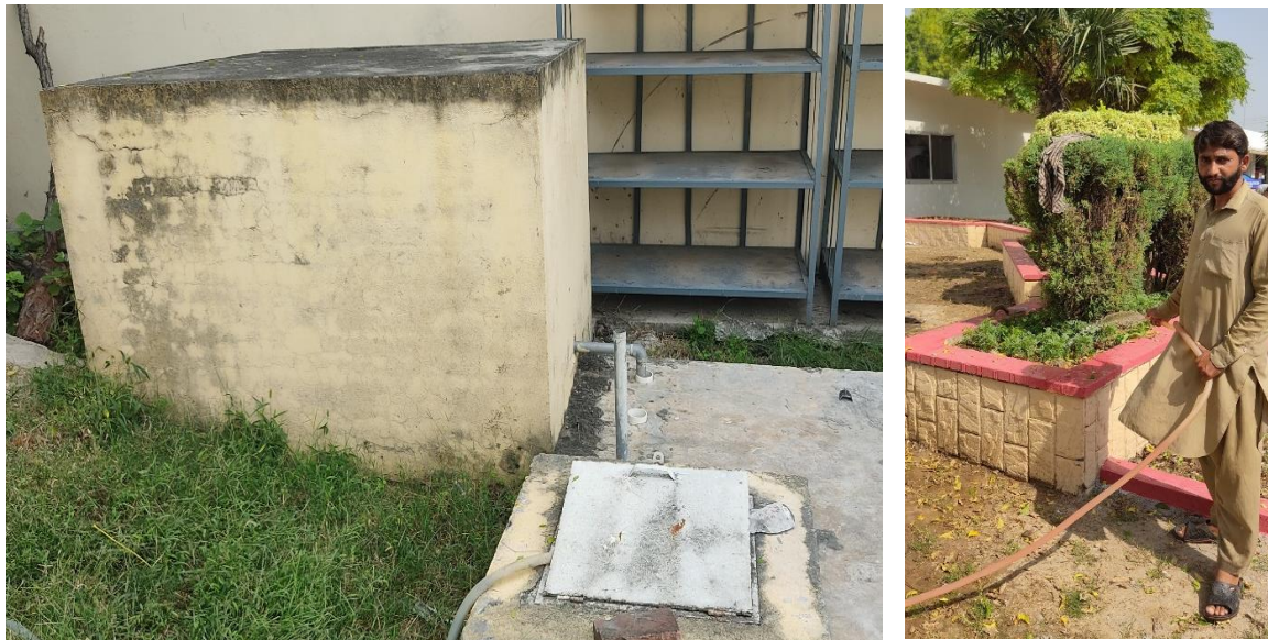
Treated water is saved in underground water tanks and is used for gardening
