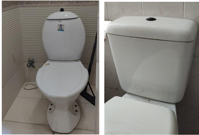
Treated water is used in toilet flush
