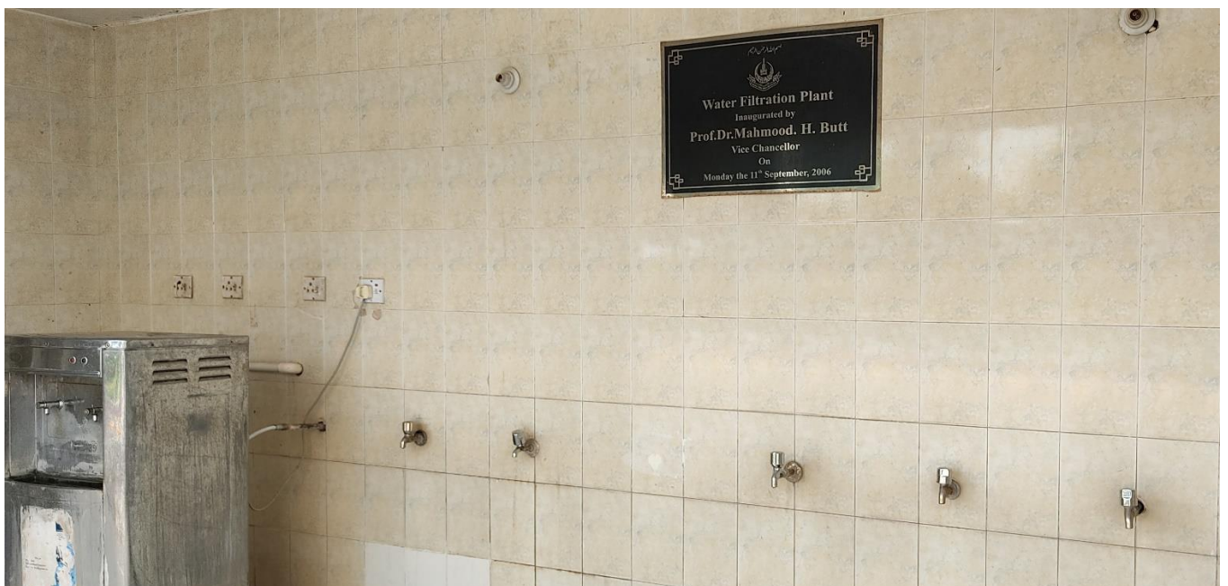
Water filtration Systems are installed. Stored water is filtered and used for drinking
