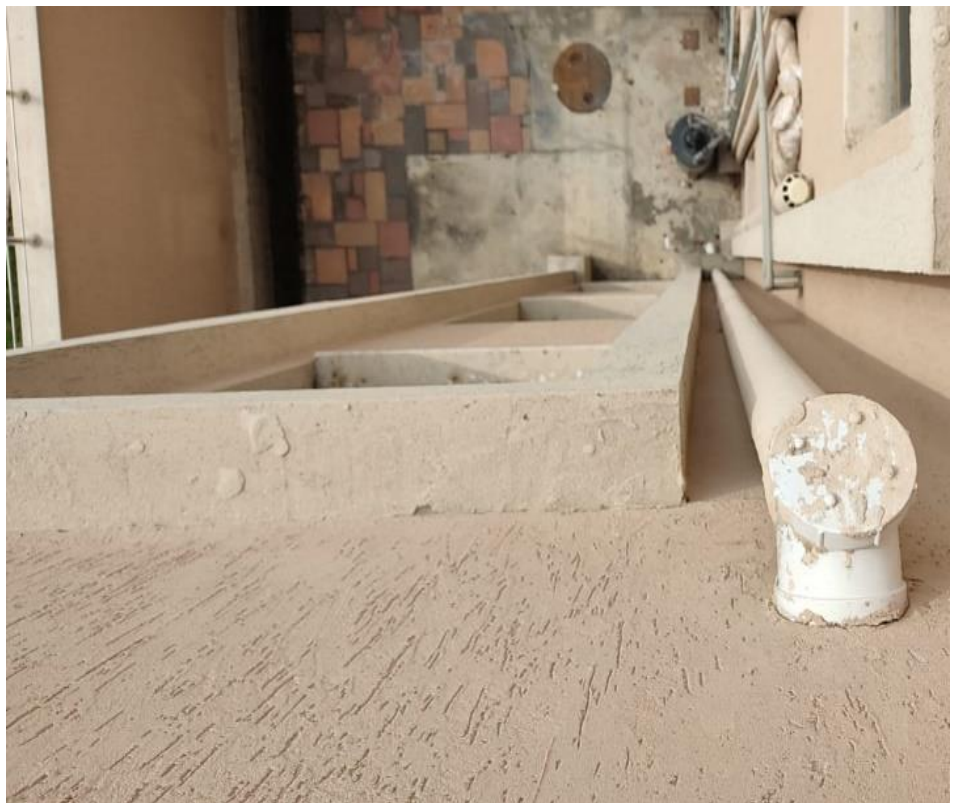
AIOU's Sewage Collection System
