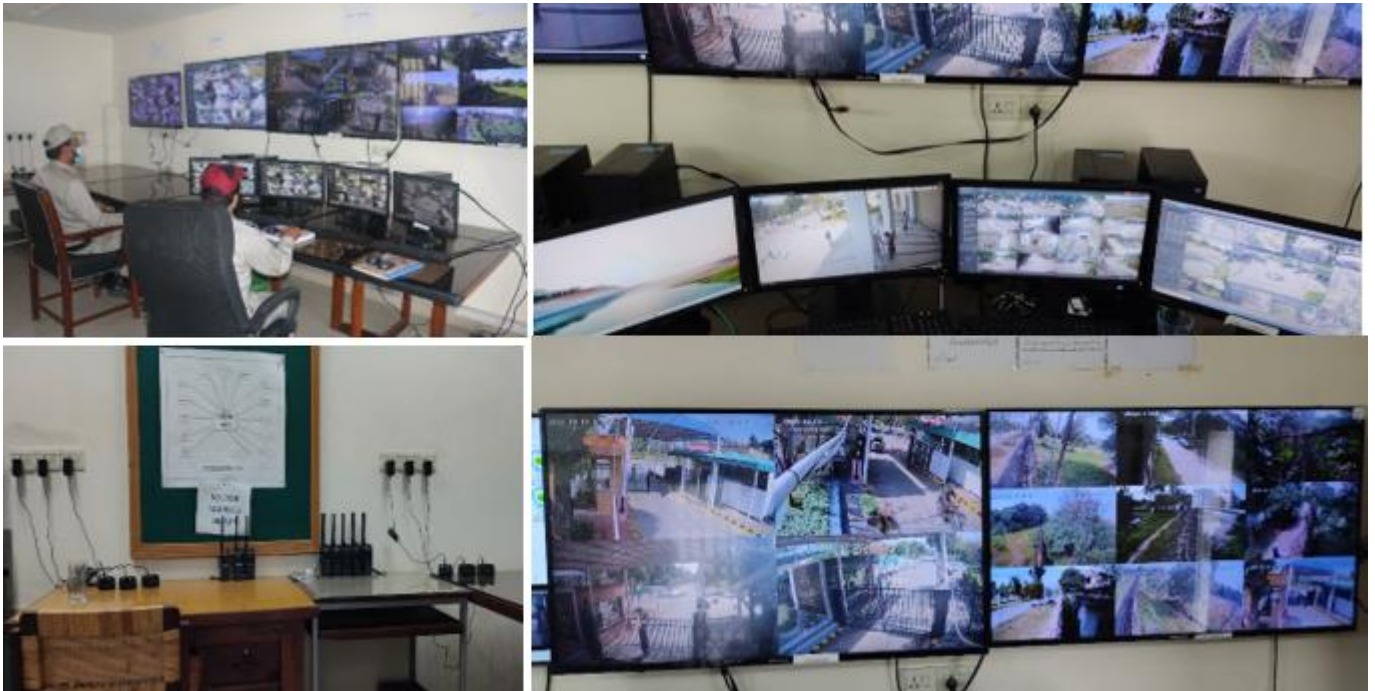
Security Control rooms
