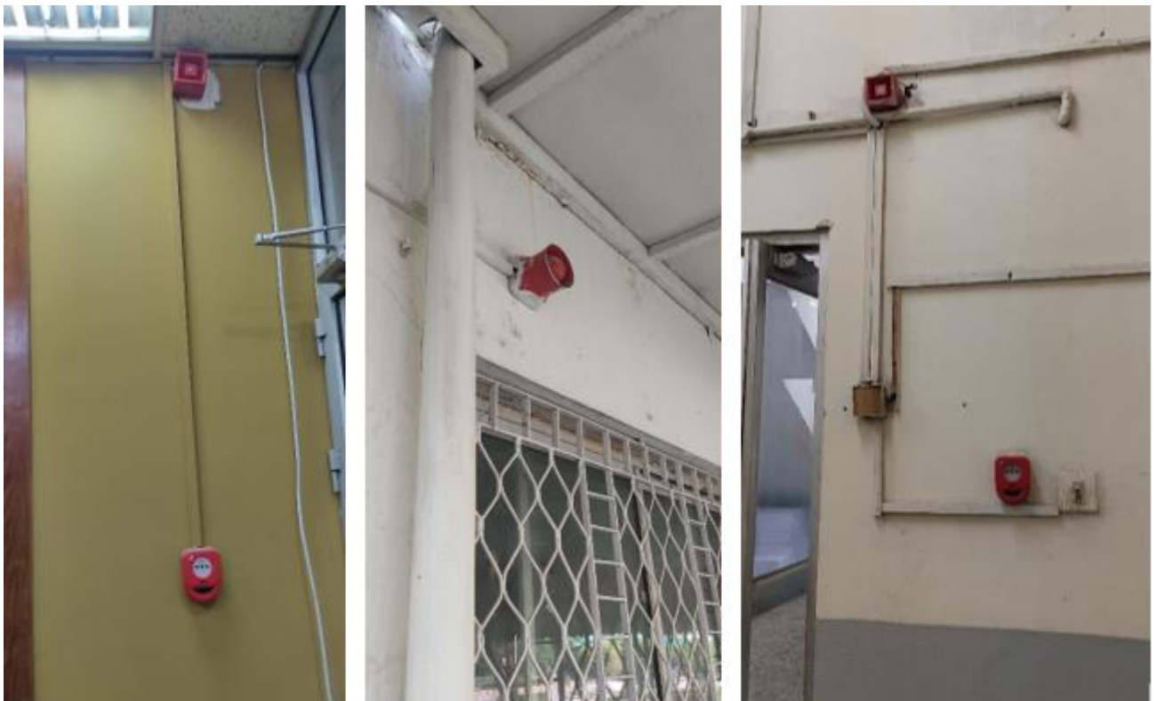
Security alarms in different buildings
