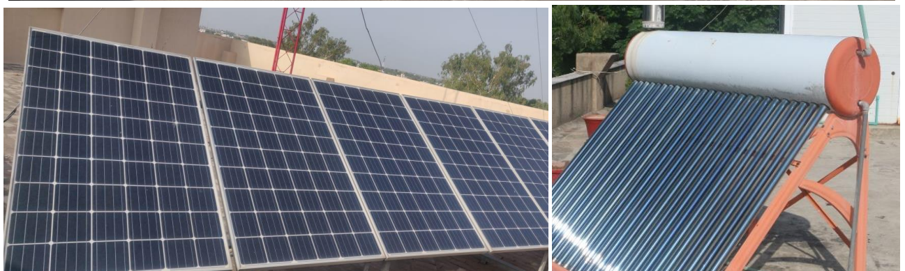
Solar Panels installed at main campus and some regional campuses
