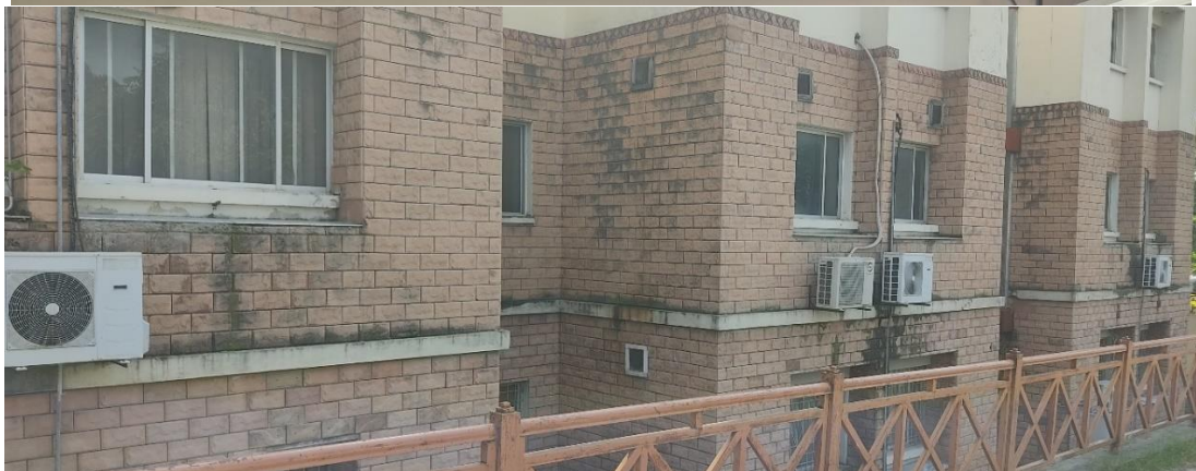
Energy efficient inverters (Combined Cooling Heating and Power Integration Unit)
