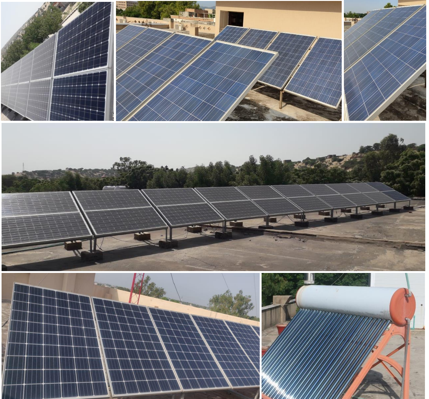
Solar Panels installed at main campus and some regional campuses
